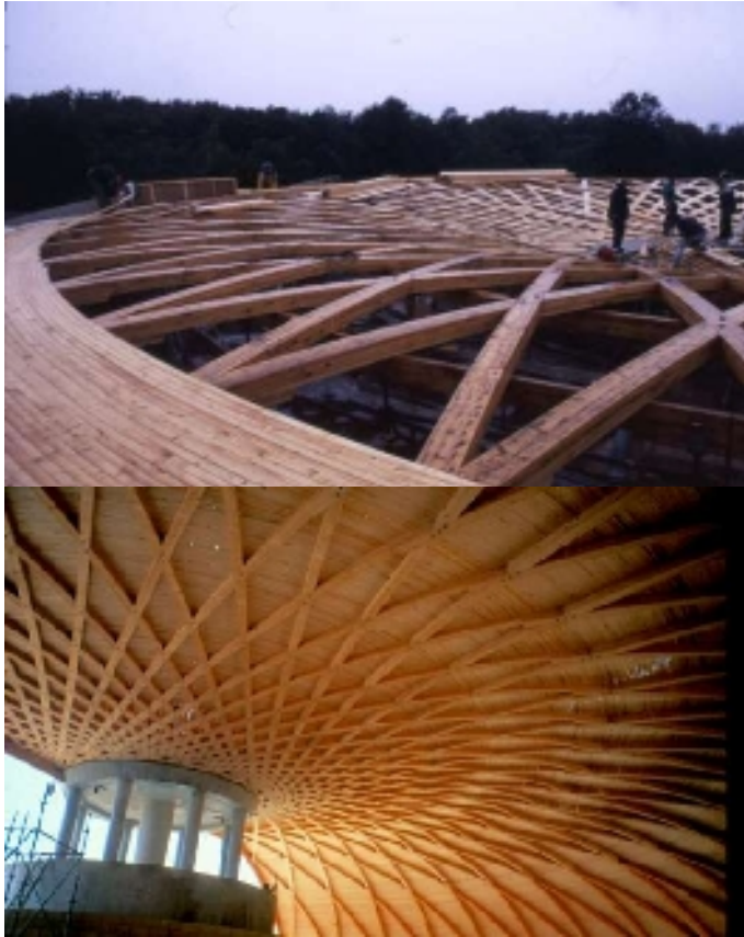
figures 36.3 and 36.4 : construction, toroidal roof composed of geodesic arcs in nailed planks allowing easy crossing at the nodes.
